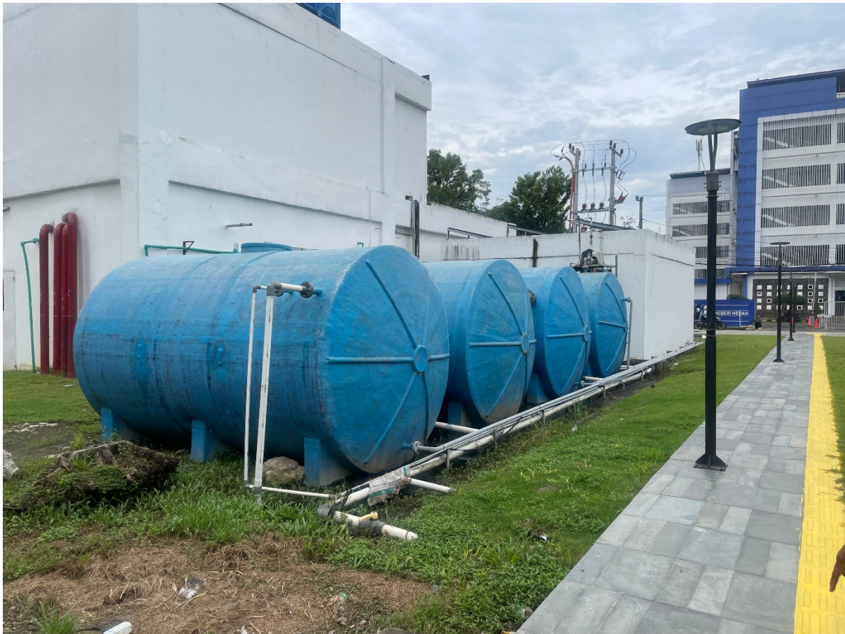
2. Waste Treatment Tank
