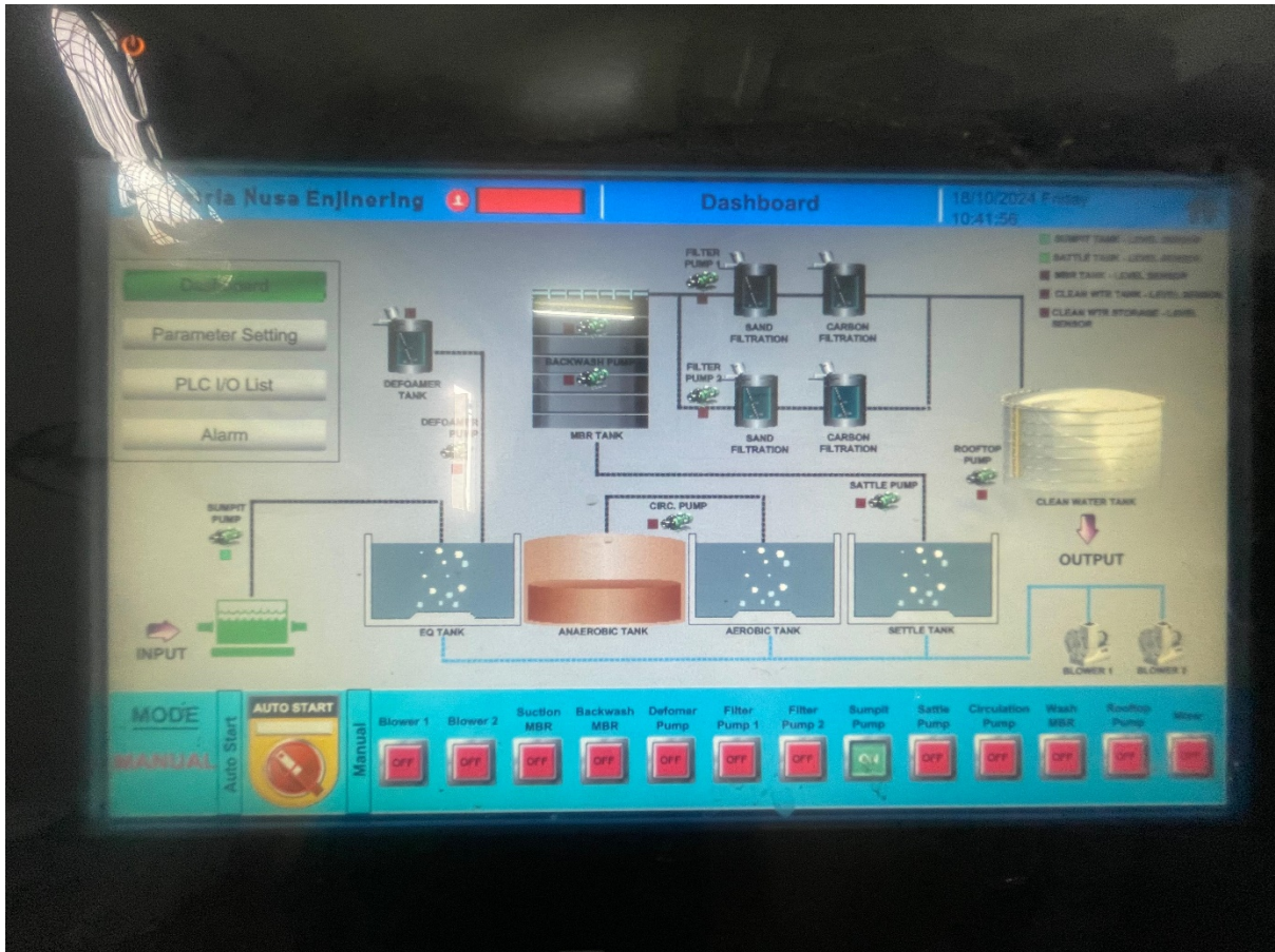
1. Wastewater Treatment Machine Control Panel
