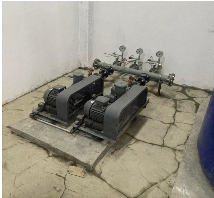
6. Water Pump Machine.
