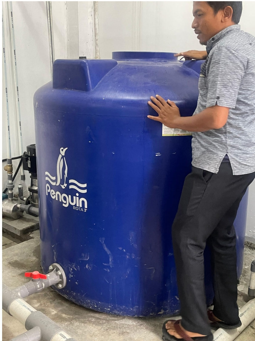
4. Neutralized Water Storage Tank.
